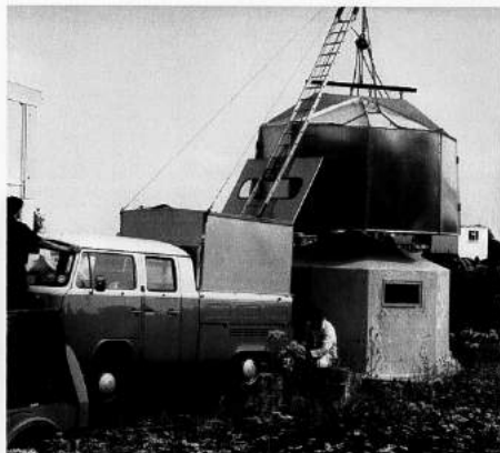
Oxfam Emergency House-Making Unit in operation following an earthquake in Lice, Turkey, 1975
