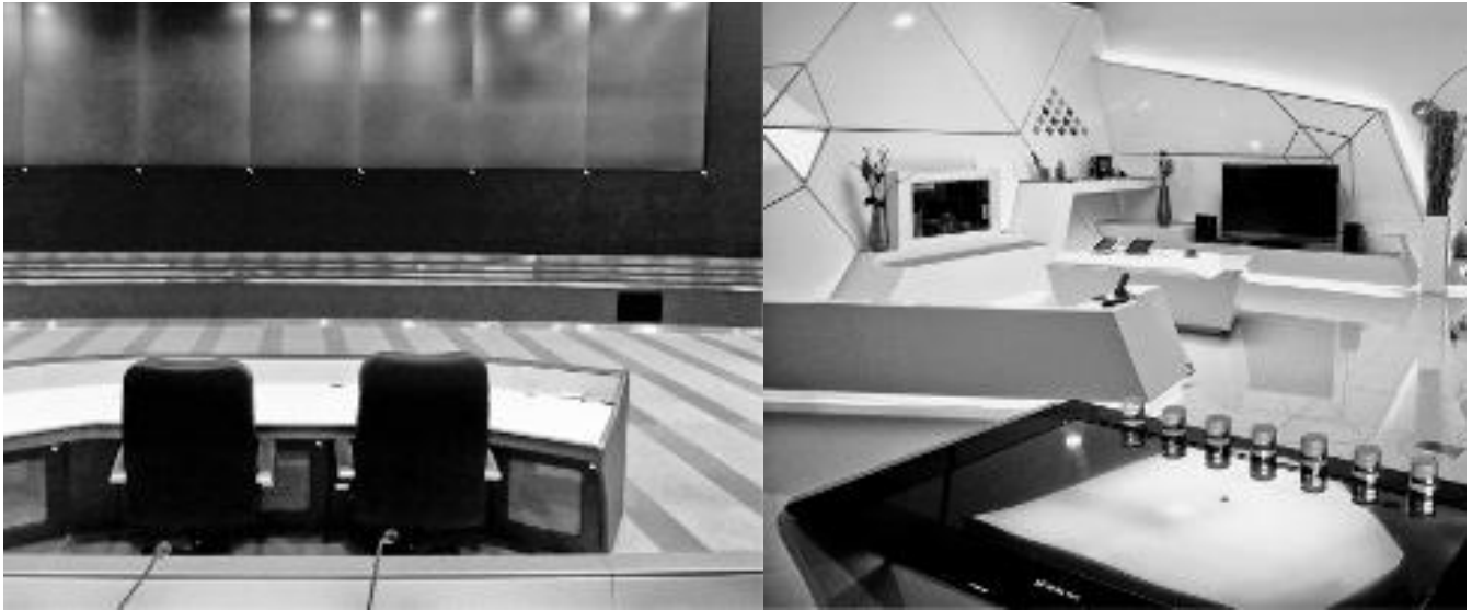
FIG. P.3__ Visible : demonstration control room, Tomorrow City, Songdo. Image: author, July 4, 2012. Ubiquitous : “smart” ubiquitous home prototype; the table and the walls are all projection-responsive interfaces, along with sensors for environmental control and telemedicine, at SK Telcom “U” (for ubiquitous) products showroom, Seoul. Image: author, July 3, 2012. Smart : “smart” pole, with sensors installed for movement detection, Internet wi-fi hotspot, surveillance cameras and sensors linked to police, fire, and hospital for emergencies, and “smart” LED screens. The poles play music to passersby, provide direct-to-consumer advertising, and enhance, according to →
